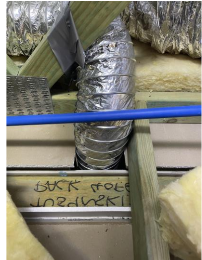
Duct through ceiling – note removed insulation
