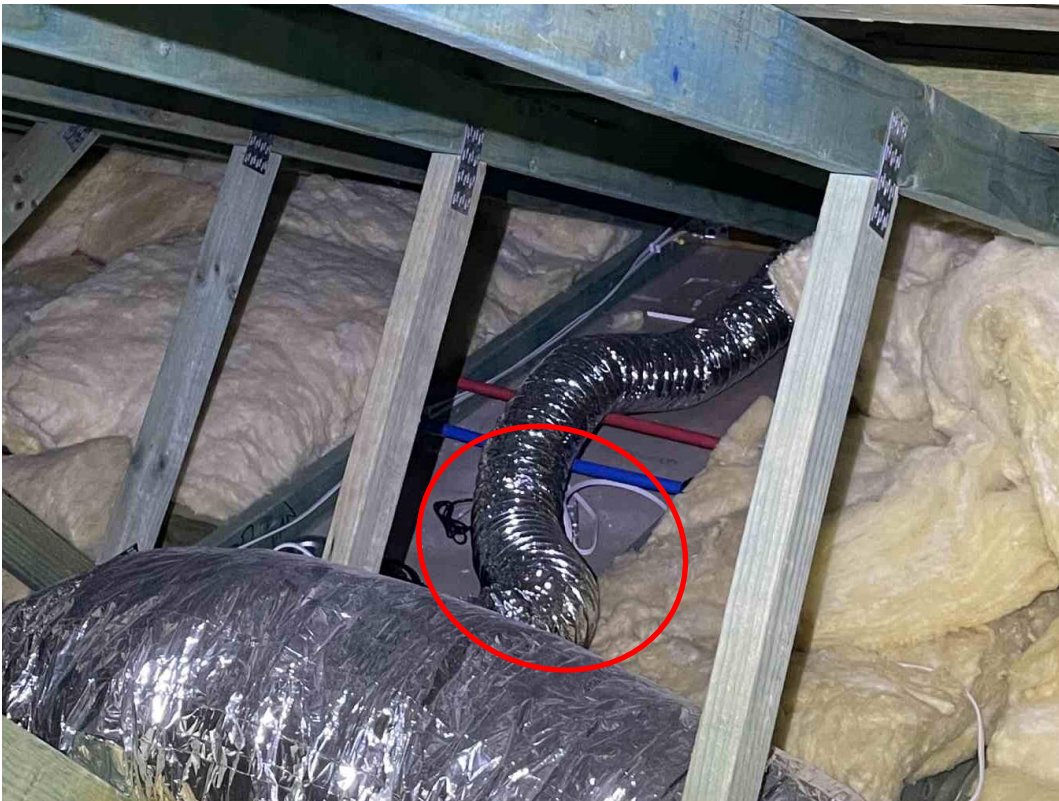
Figure 34 Crimped excess exhaust fan ductwork
