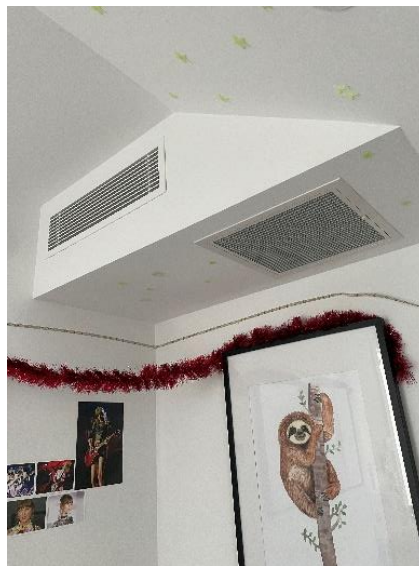
Bulkhead over bed, where dust collected during testing
