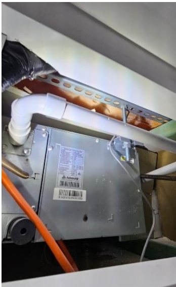
Insulation visible above unit, showing poor isolation
