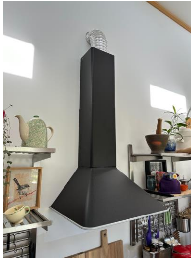
Ducted through wall
