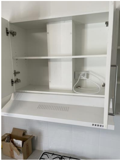
Typical kitchen rangehood
